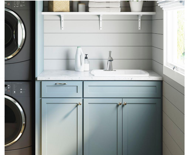
The utility sink for washing will also enjoy a second life as a hand-wash station, perhaps with motion sensor plumbing fixtures for touchless use. (PHOTO: Sterling Plumbing)
